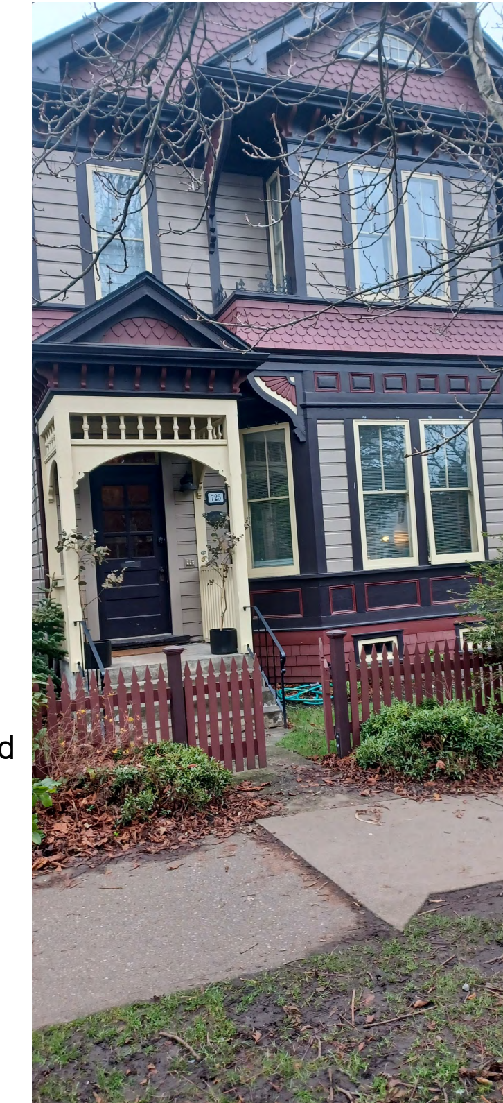
Douglas Fir heritage door installed within the sunken courtyard will match existing colours of main front door
