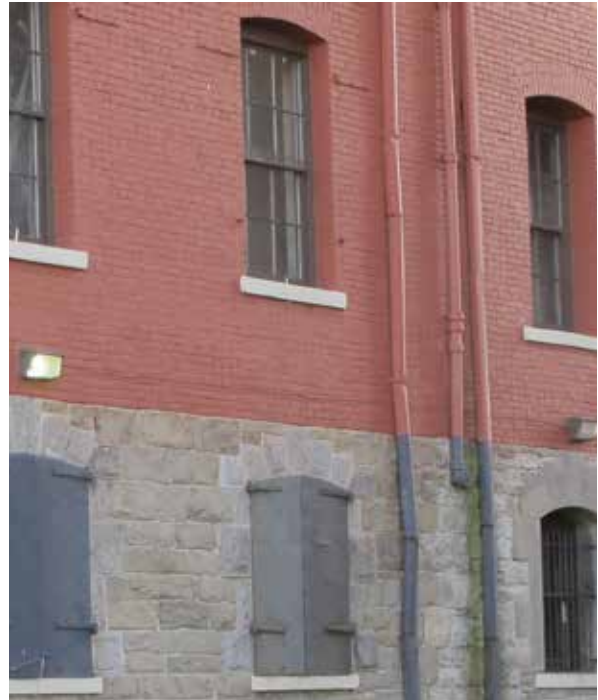
Above: 6-over-6, hung, wood windows on rear elevation. Note fire shutters present at lower level and evidence of past shutters on floor above.
