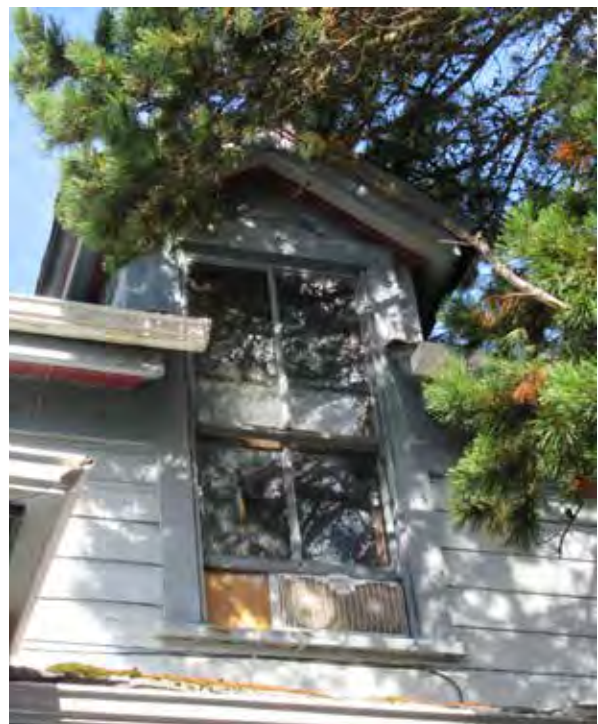
Above: Original two-over-two wood assembly hung window of upper level (top) and gabled dormer (bottom) with integral sash horns.
