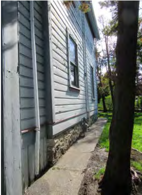
Above: Field stone foundation of west facade. Note presence vertical wood siding at foundation at rear of residence.
