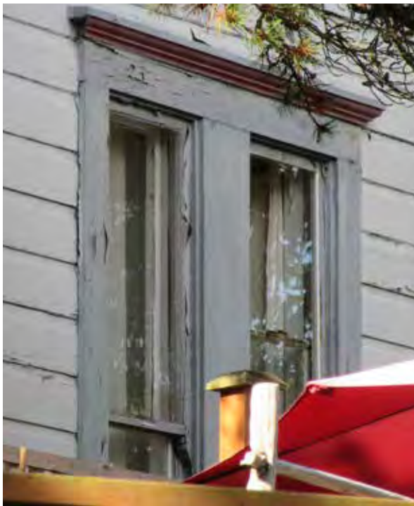
Above: Original double assembly one-over-one hung wood windows with integral sash horns on east elevation.
