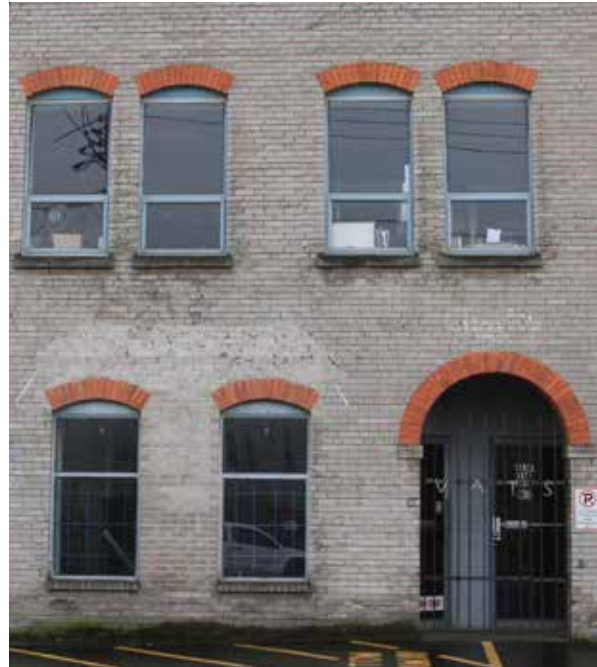
Above: Fenestration of front elevation with replacement window and door assemblies. Original openings, sills, and lintels remain intact, with exception of ground floor windows.
