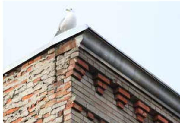
Above: Original metal cornice of front facade and later added cap flashing.
