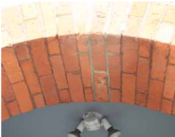
Top: Previously restored area of first floor front façade. Note crack in brick, difference in mortar and brick between original and restored section, and epoxy residue on brick.
