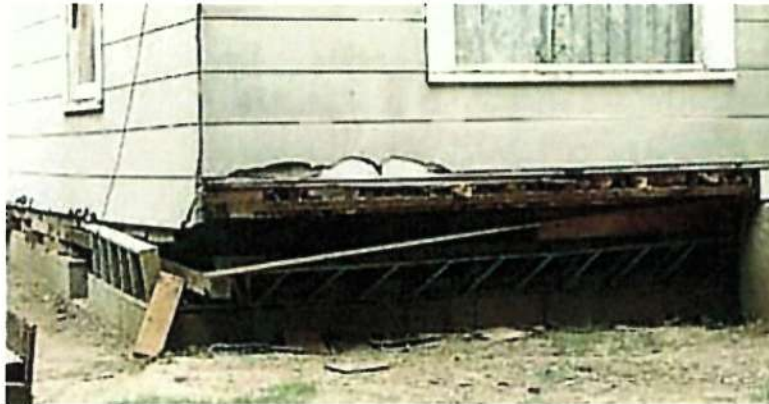
Figure 15: Cripple Wall Failure Due to an Earthquake (homerepair.com)
